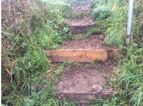
A collapsed riser on the steps on FP7 at the bottom of Church Field was replaced
